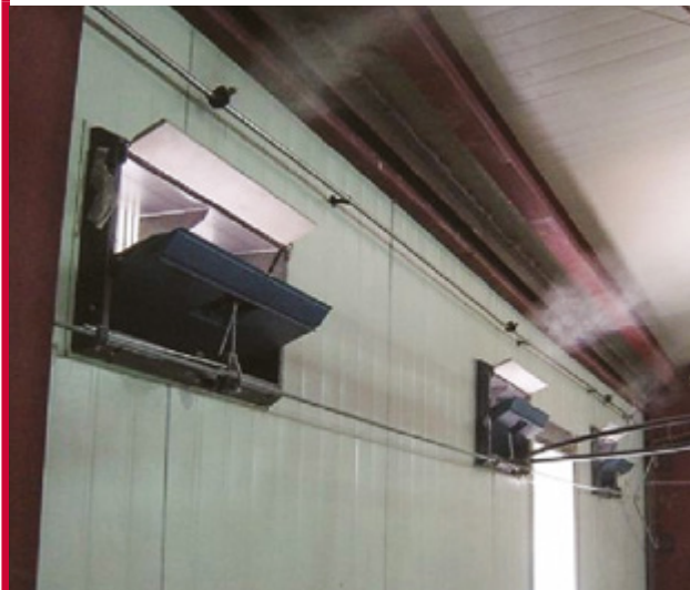
Figure 112 Example fogging system for a cross-ventilated house.
