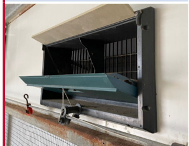
Figure 100 Example of a good-quality air inlet.
