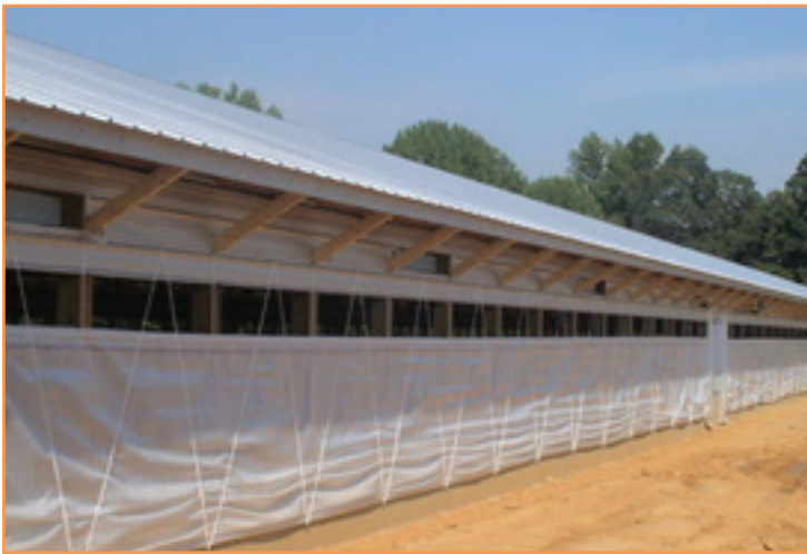
Figure 3: Example of a roof painted white to help reduce the heat load for the house.
